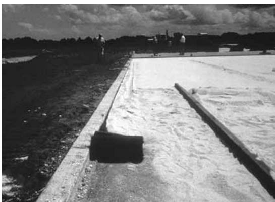
Figure 7. Woven geotextile used to contain bedding sand from migrating laterally. Visit < www.icpi.org > for detail drawings.
